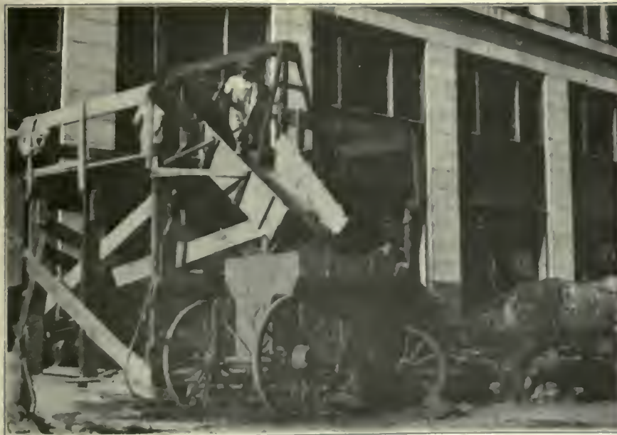
FIG. 48. BUILDING OPERATIONS, A SOURCE OF DUST. During the construction of large buildings or in the wrecking of old ones, the refuse is frequently handled by chutes. This method provides excellent opportunity for the wind to blow away large quantities of dust.
